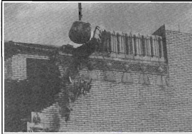
Masonic Temple (top) stood on Fourth Avenue from 1920s to 1975 when torn down to make way for Federal Building. The temple, built to last, withstood the first few strikes of the wrecker's ball unfazed, but ultimately the ball won (lower picture).
